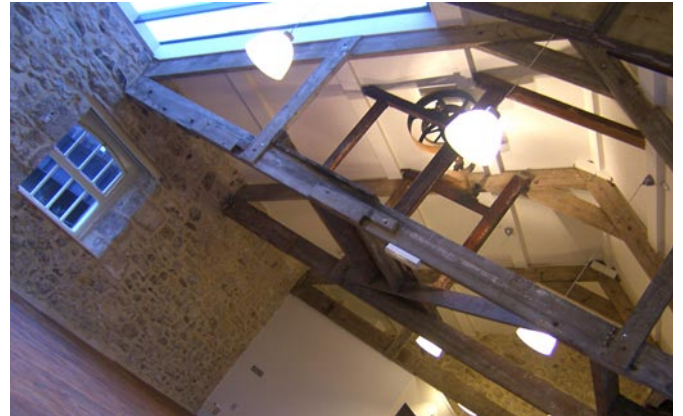
White's Warehouse in Foundry Square, Hayle which has received investment from Objective One via Penwith District Council's Hayle Townscape Heritage Initiative
